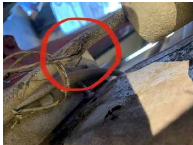
Picture1. Damaged cable
